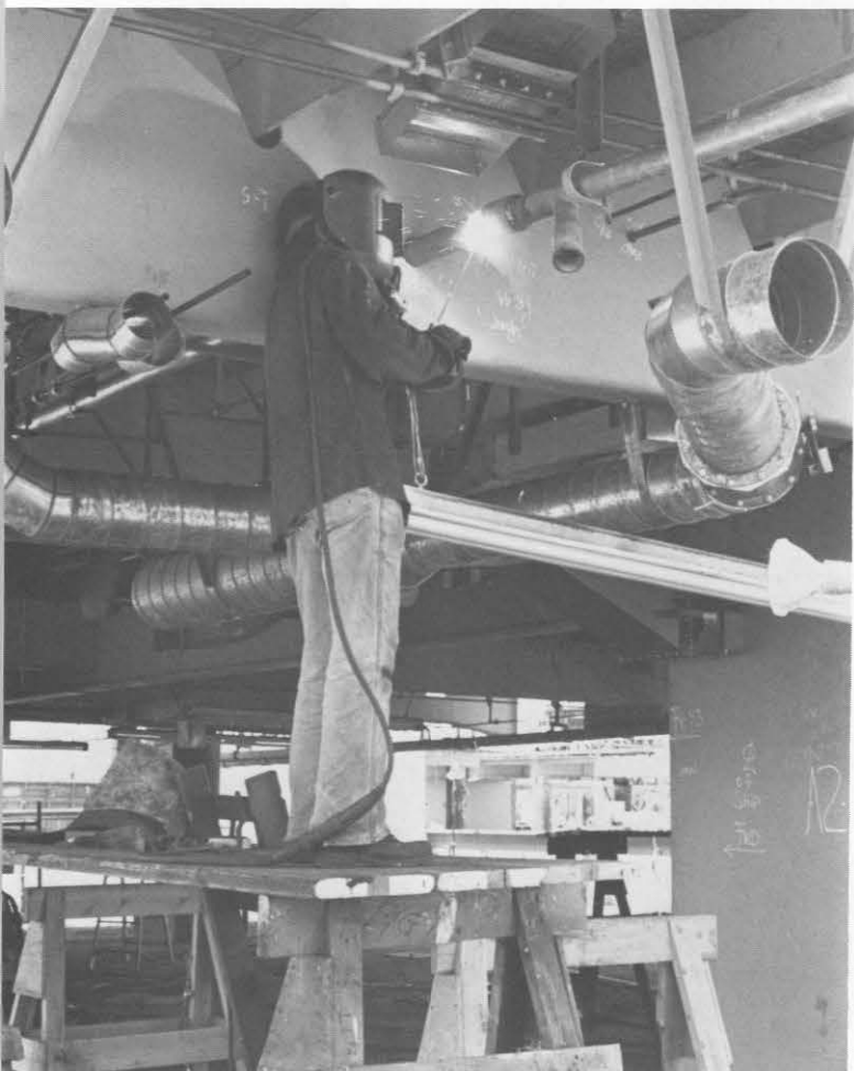
A pipe welder performs last-minute preparations to a unit prior to its erection.
